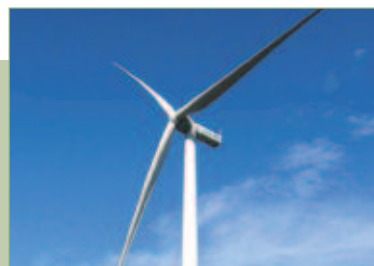
Wind Turbine System
