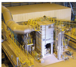
取鍋精錬炉 Ladle Refining Furnace
